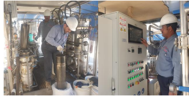
Transformer Corrosive Sulphur Treatment
