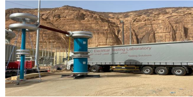
Onsite High Voltage Testing system
