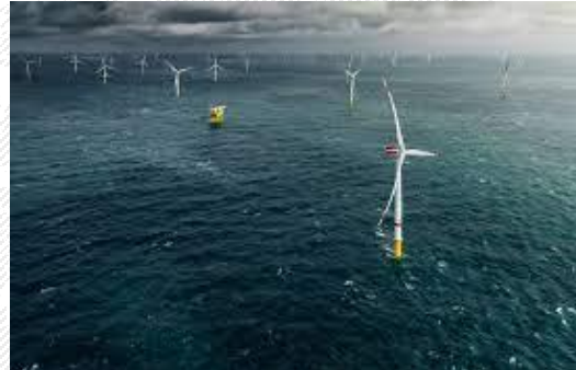
Inter-array cable offshore wind park Baltic Eagle – 66kV 2021, Germany Client: Van Oord
