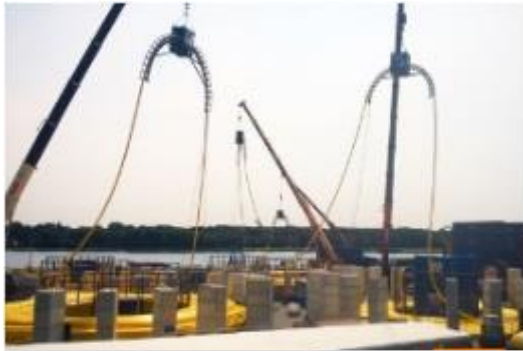
Inter-array cable offshore wind park Hohe See – 33kV 2018, Germany Client: EnBW
